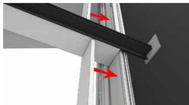
14 Use internal foamboards to space out rafter positions before fixing rafters to the ringbeam.
